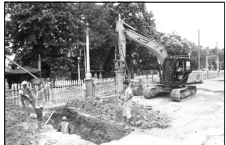
Excavation work going on near BBD Bag Mini Bus Stand adjacent to Lalidighi to identify the location of underground public utilities such as cables of CESC & Telecommunication and pipelines of water and sewerage so that these public utilities can be shifted properly. The excavation is part of construction work for Mahakaran Station of East West Metro.
