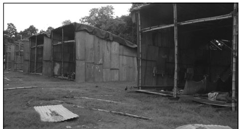
Makeshiji stalls in the process of being constructed to enable the "Baji Bazaar" in the city head of Kali Puja - Arjiji Ganuly
