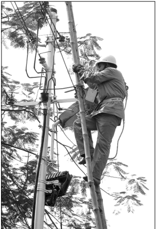
To ensure reliability of power supply during the examination season CESC has undertaken a special inspection of overhead wires in some areas. —Arjit Ganguly
