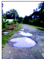
Picture shows massive potholes on the national highway road stretch near STS office, Rangat in Middle Andaman. Despite hardships being faced by commuters, repair and maintenance of the road network by concerned agencies in the government remains far from ensured. (Pic: SUBRATA)
